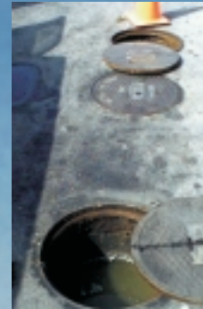
Use of an in-ground grease interceptor prevents grease, oil and fat from reaching Santa Monica Bay.
