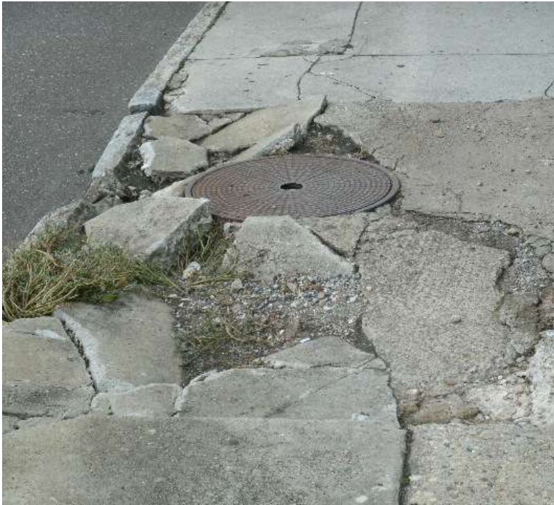
Unsafe Walking Conditions
